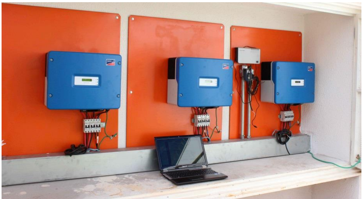
Figura 4 – Inversor Grid Tie
